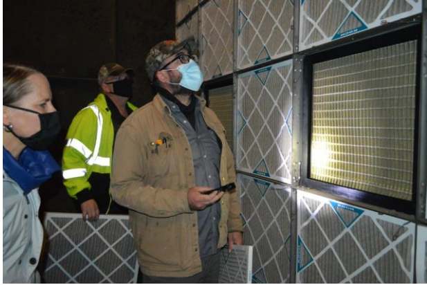
Duane and Jimmy removing the prefilter-MERV 8 to assess the MERV 14 filter for building health and safety
