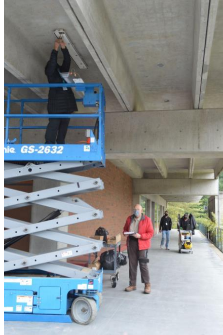
Diana and Roger install LED lighting and remove ballasts at the Sylvania campus
