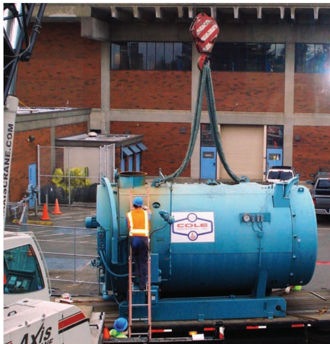
Removing an old boiler from the Sylvania campus, to make room for more efficient equipment.
