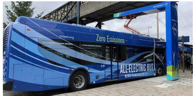
Example of existing TriMet fleet charging infrastructure at Sunset Transit Center
