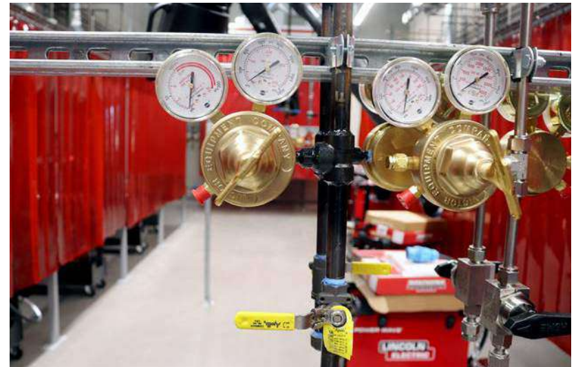
Columbia County Center OMIC welding shop
