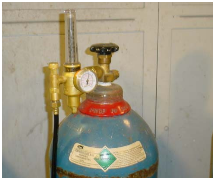
Cylinder with flow meter
