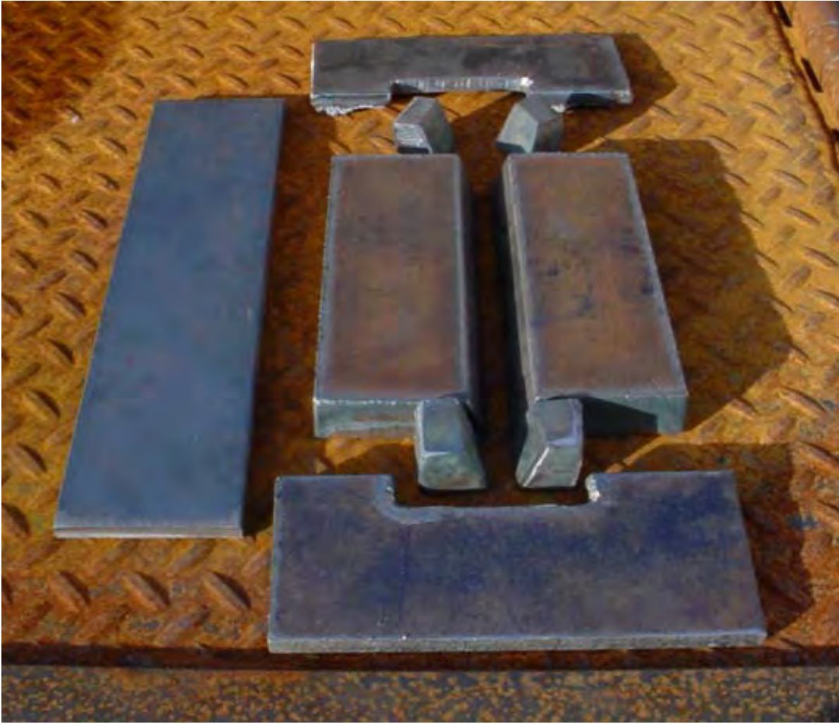
All the pieces to assemble a Single V Groove Weld with Strong Backs.
