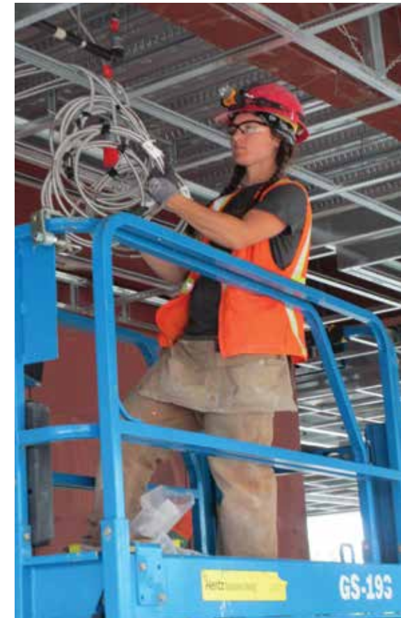
Above: JoceyIn Atkins of Cherry City Electric works on the new addition for Building 5, the campus hub.
