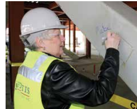
Above: To celebrate the progress of construction at Building 5, a beam signing ceremony was held in February 2015. Sandra Fowler-Hill, president of Rock Creek Campus, leaves her mark for posterity on the designated brace.
