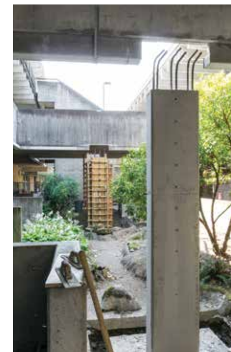
Left: Additional seismic upgrades, such as new bridge foundations to allow individual building movement in the event of an earthquake, are all part of the master upgrade plan for the Sylvania Campus structures.
