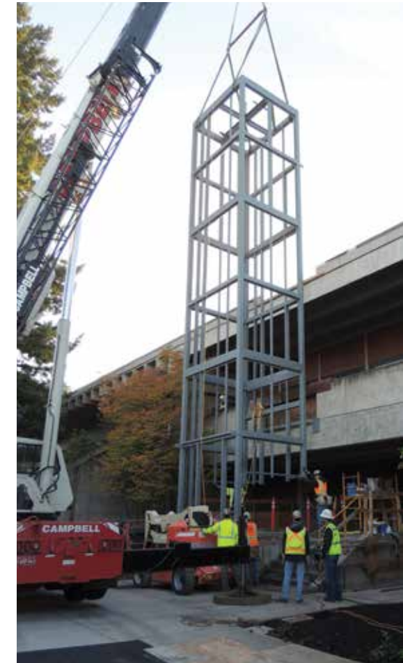
Above: Completed in December 2013, the new glass elevator at the north entrance of the CC greatly facilitates ADA access to all levels of the building, including roof access for efficient maintenance of the mechanical systems.
