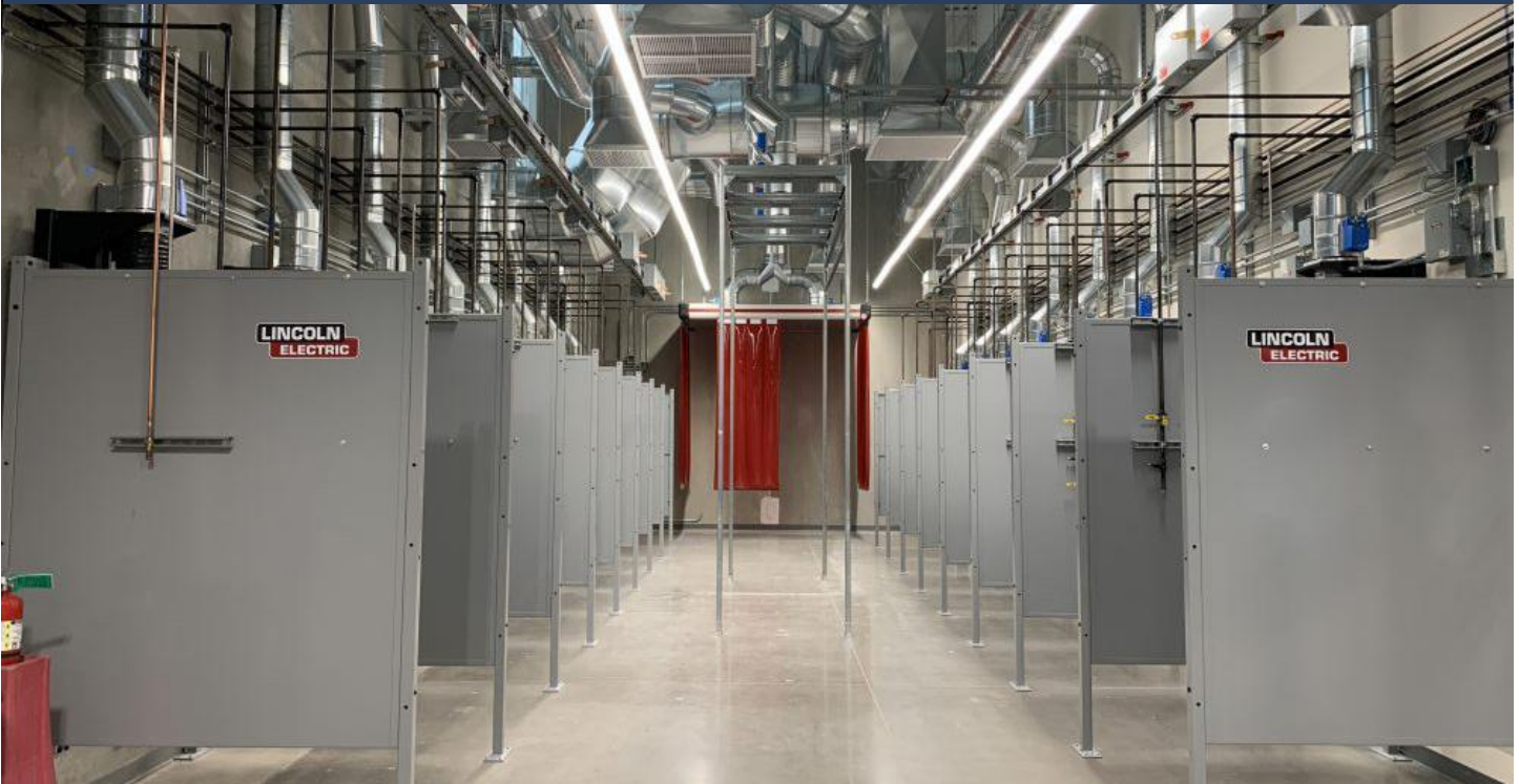
BELOW: Welding stations inside the newly constructed Oregon Manufacturing Innovation Center Research and Development (OMIC R&D) in Columbia County
